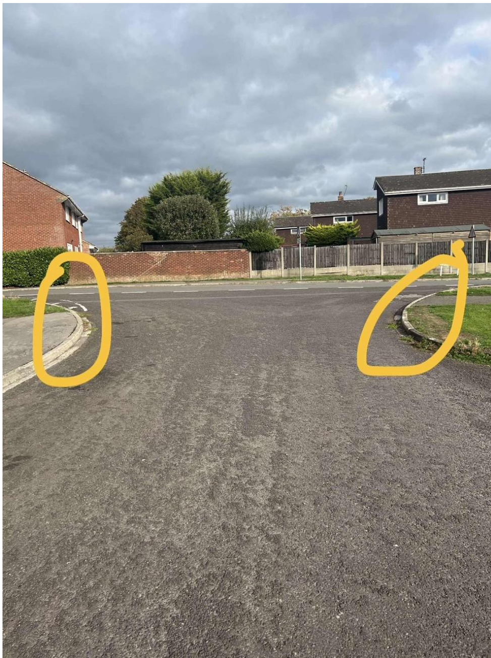
Resident photo of kerb on Trenchard Way
